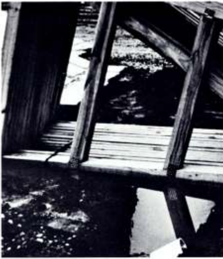
Trusses may gain moisture and swell if they are allowed to lie in water at the job site.
